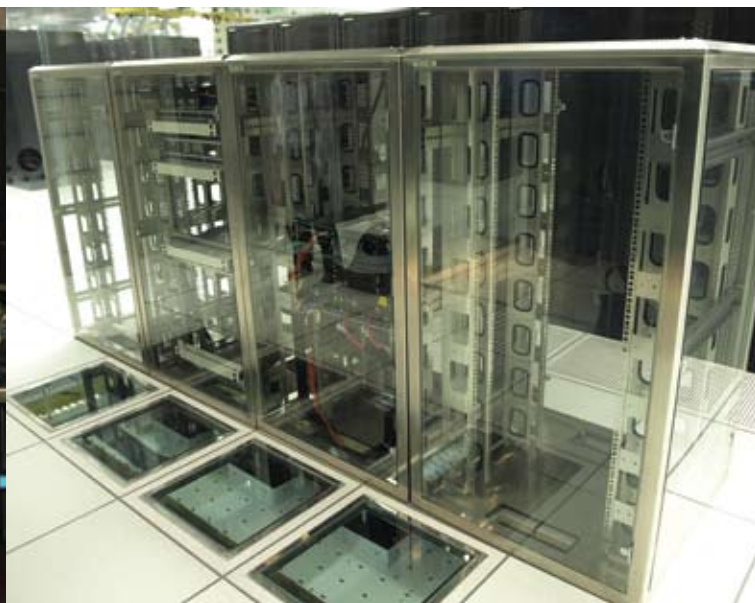
The server rack that houses the MyIX exchange
