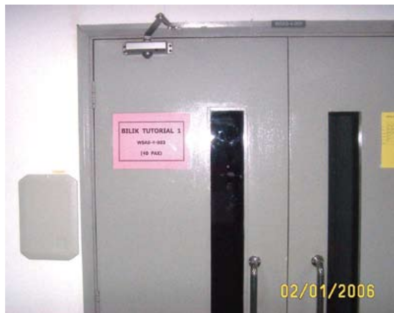
RFID Access Control
